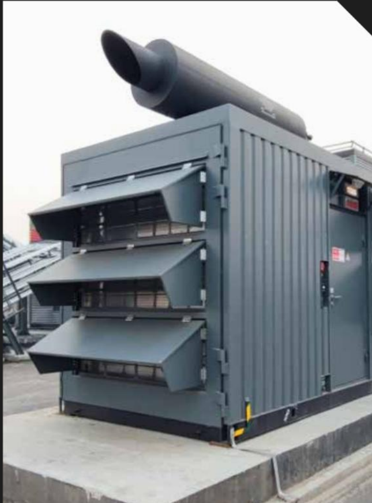
Diesel gensets 柴油发电机组
