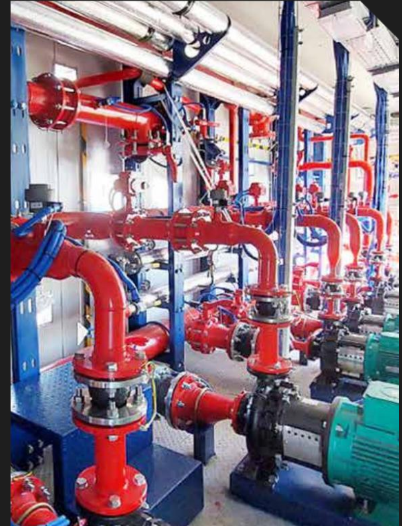
Block pumping stations
