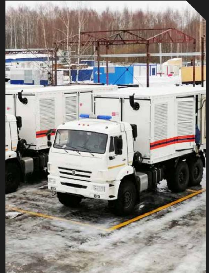
8.5 MW portable electric power plant for Rosseti
