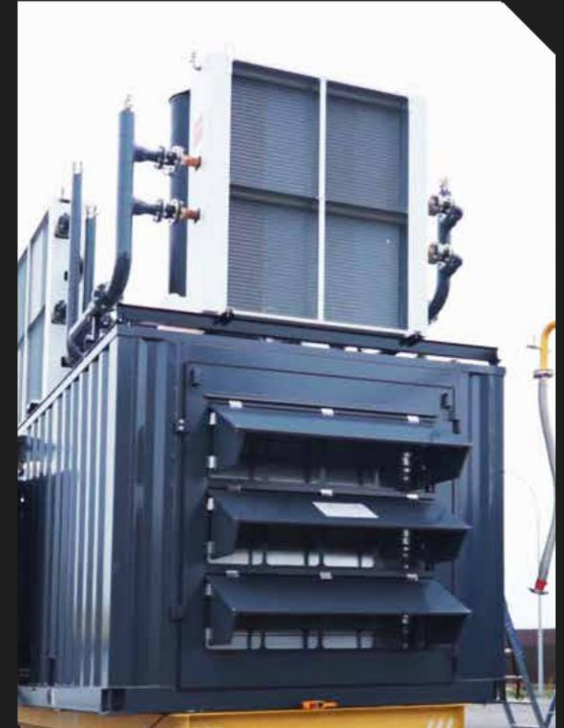
1MW gas-fired power plant for glass factory
