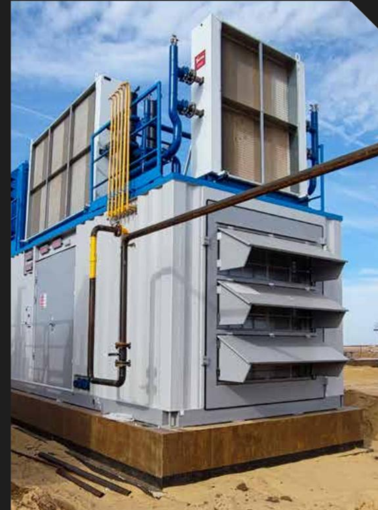
3.5 MW gas-fired power plants for Gazprom
