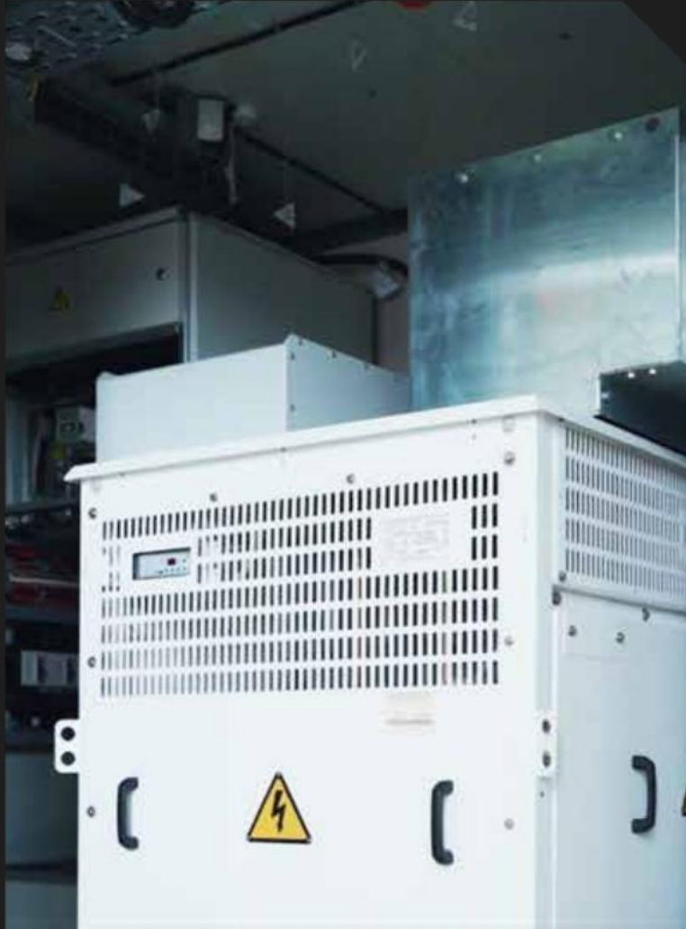
Complete transformer substations 集成电源
