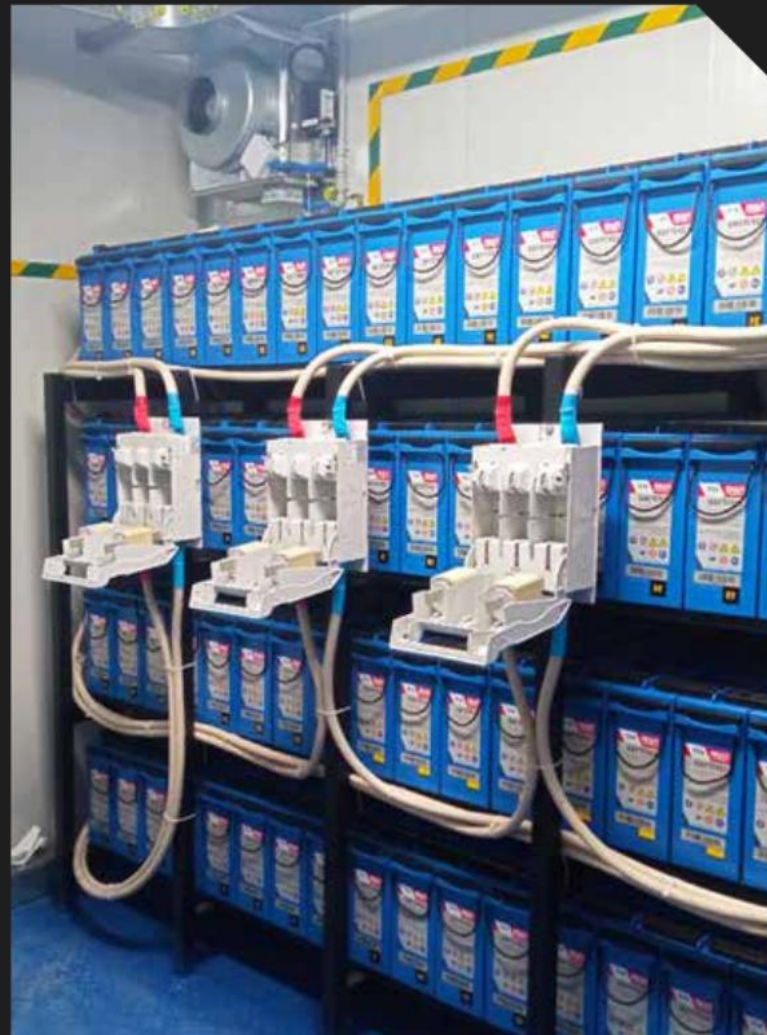
Uninterruptible power supply 不间断电源
