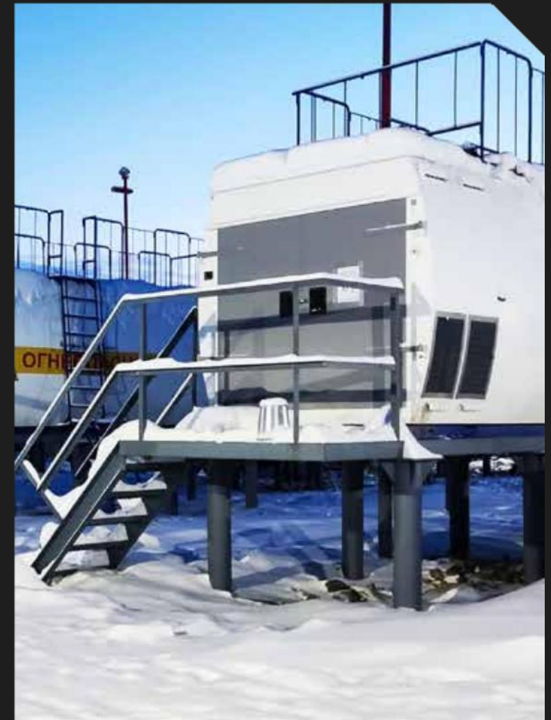
Fuel storage tanks 燃料储罐
