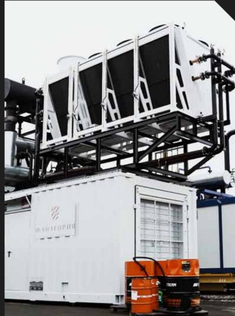
1MW gas-fired power plant for Fanagoria winery
