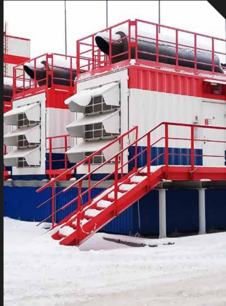
9 MW diesel power plant for NOVATEK-Murmansk
